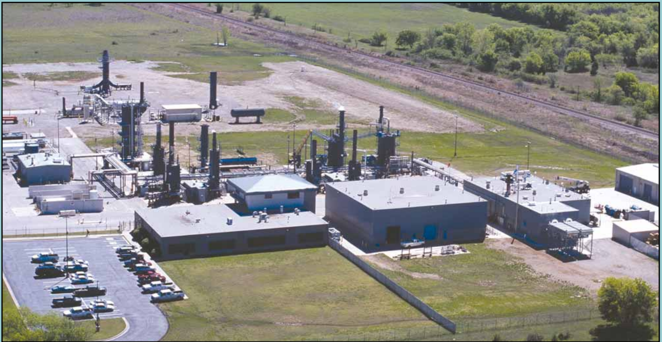
John Zink Company's Research and Development Test Center is located on the campus of the company's world headquarters in Tulsa, Oklahoma.
